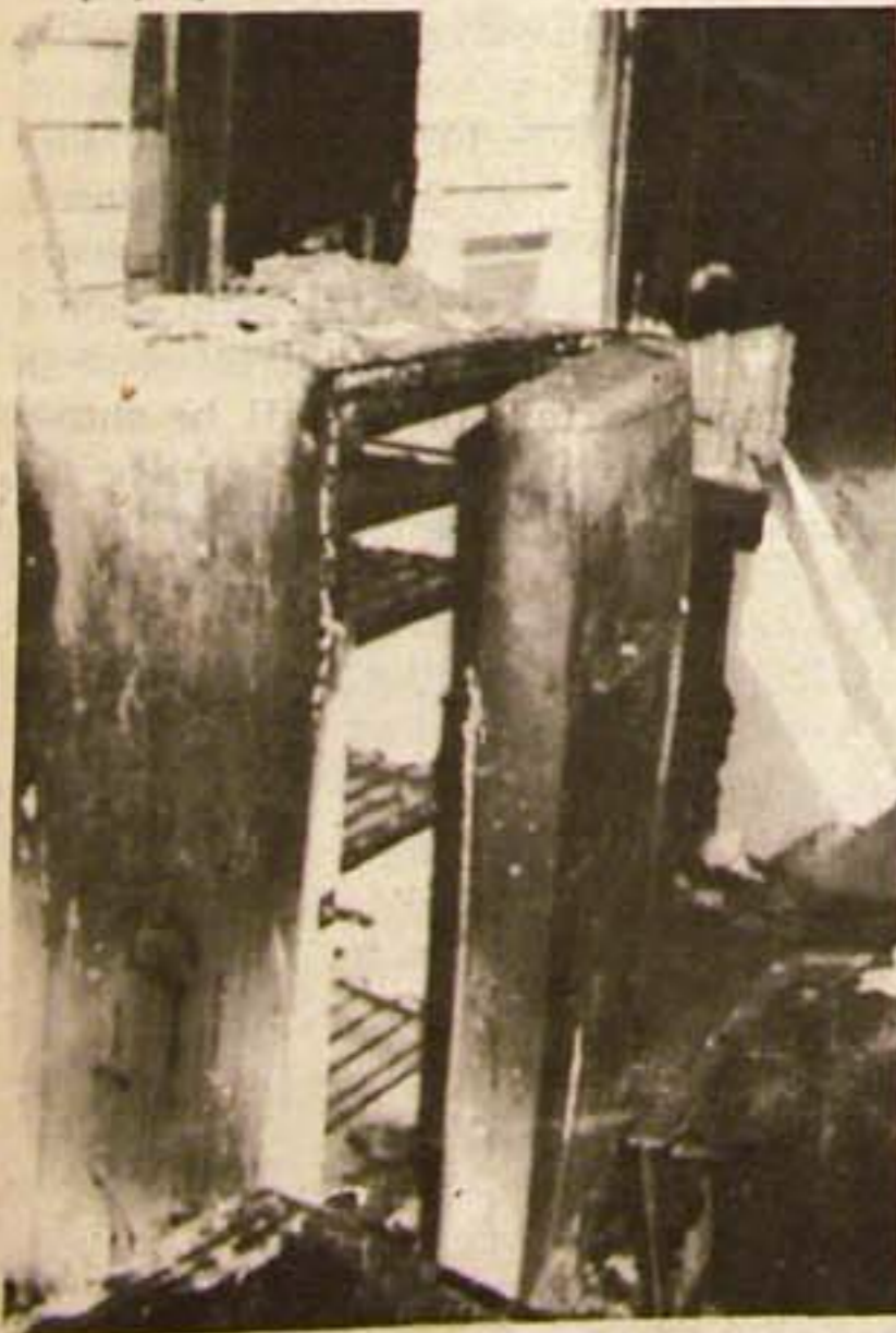
Inside of burned home
